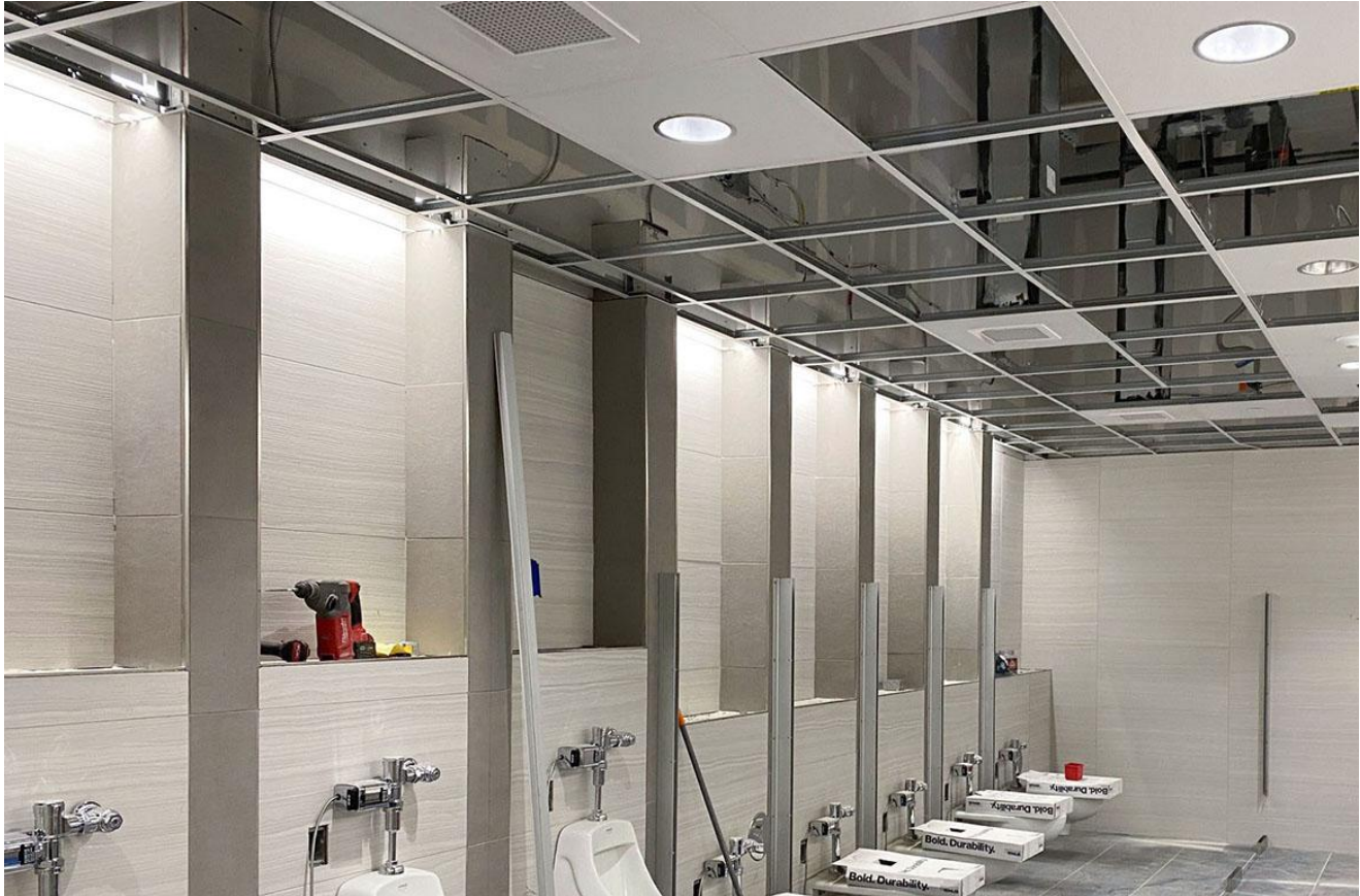
Tile installation at the Texas Facilities Commission, North Austin Complex Phase One project
