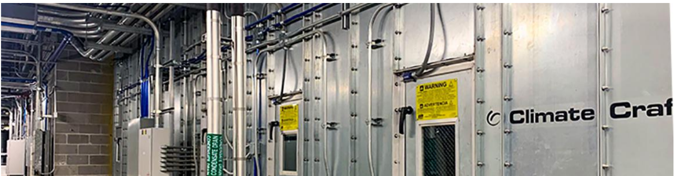
Air handling unit (AHU) equipment installation at the University of Texas Health Science Center at Houston, Medical School Building Penthouse AHU Replacement project.
